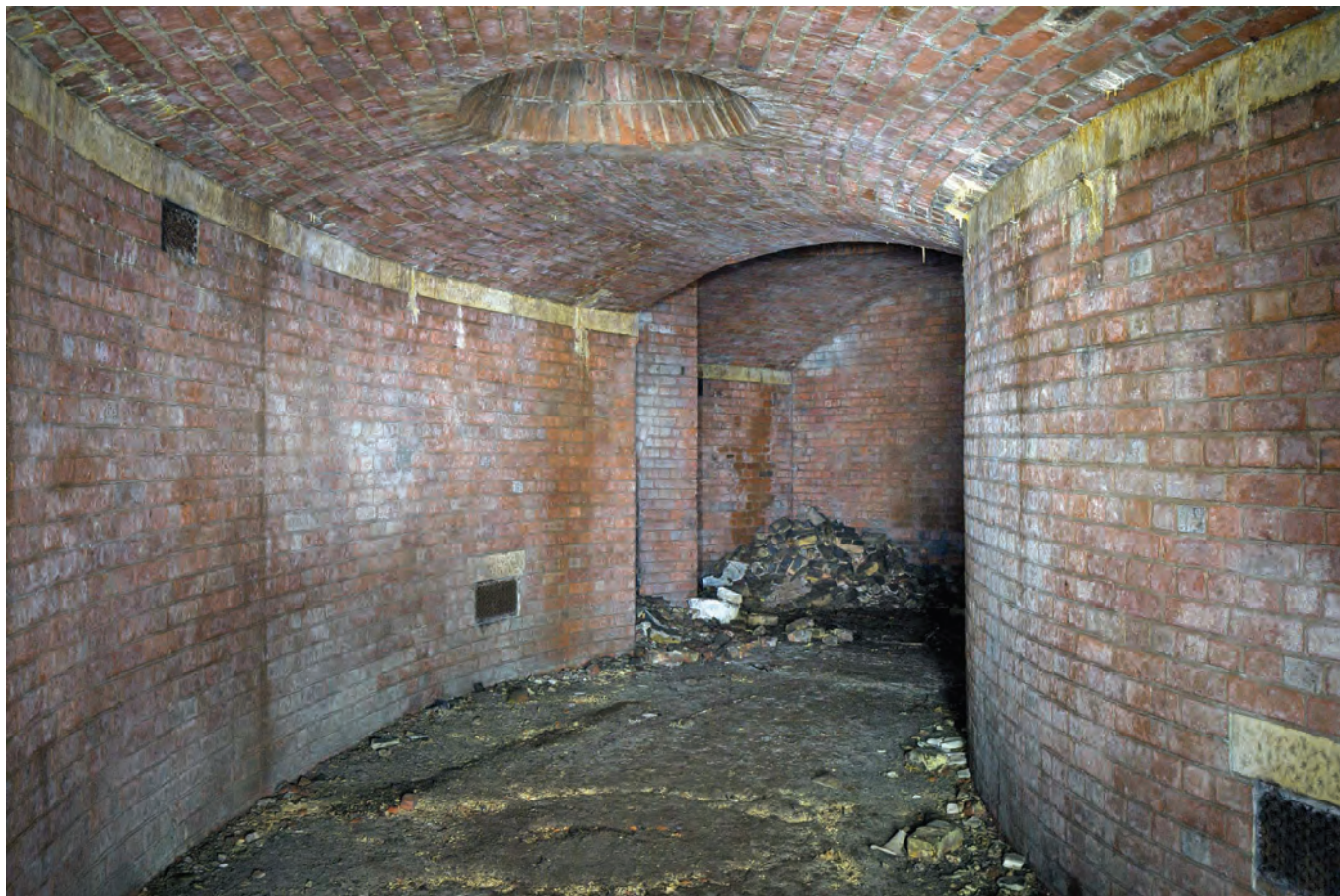
The only section of the sprawling tunnel system in the grounds of Welbeck Abbey to remain easily accessible is a short spur tunnel built for a purpose unknown. Note the skylight in the roof. Photo Ben Walker
